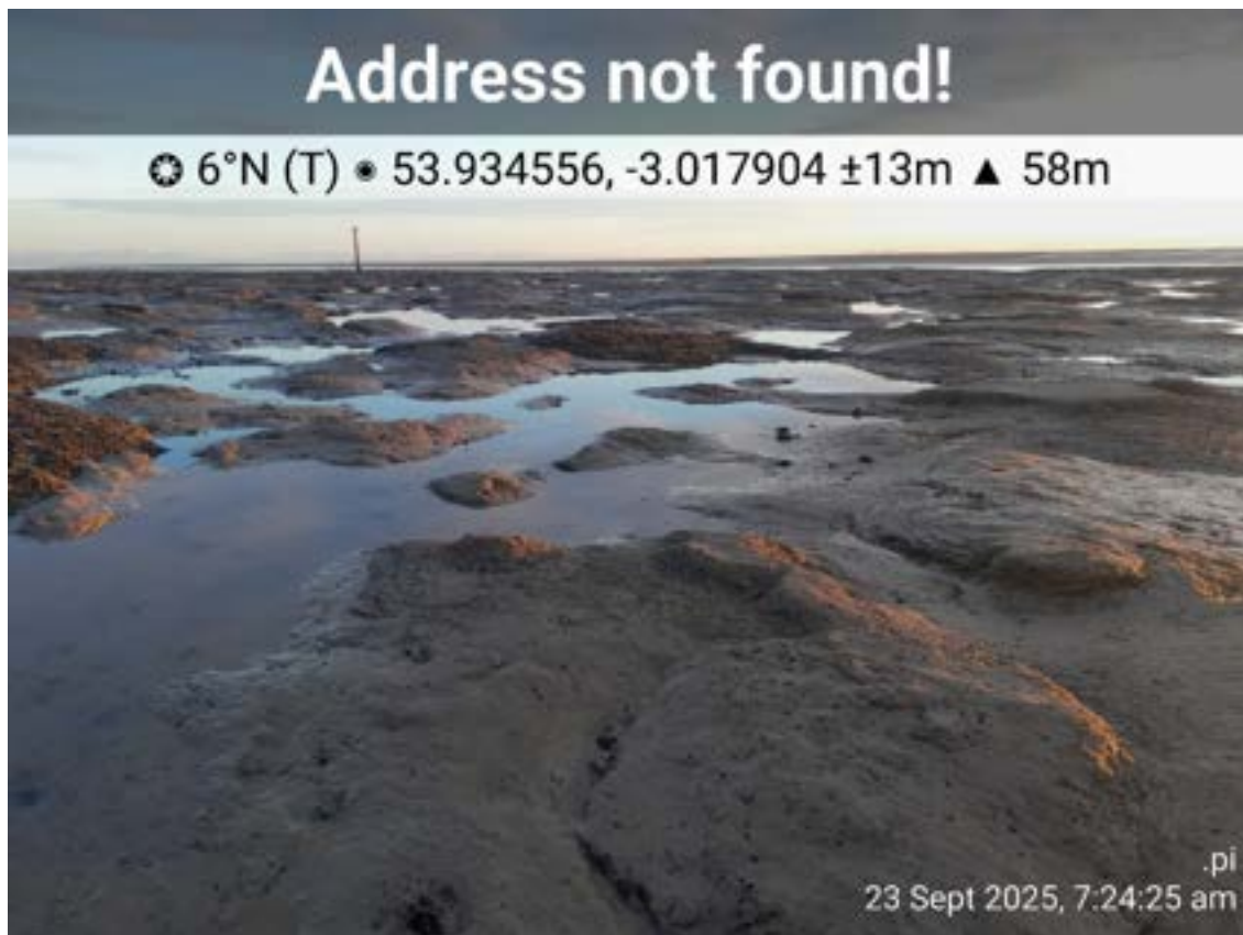
Image 1. Evidence of scour on Black scar
